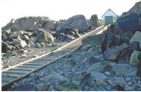
Maritime Construction and Engineering LLC, of Cape Neddick, this month completed the repair of the Nubble Light boat ramp.
